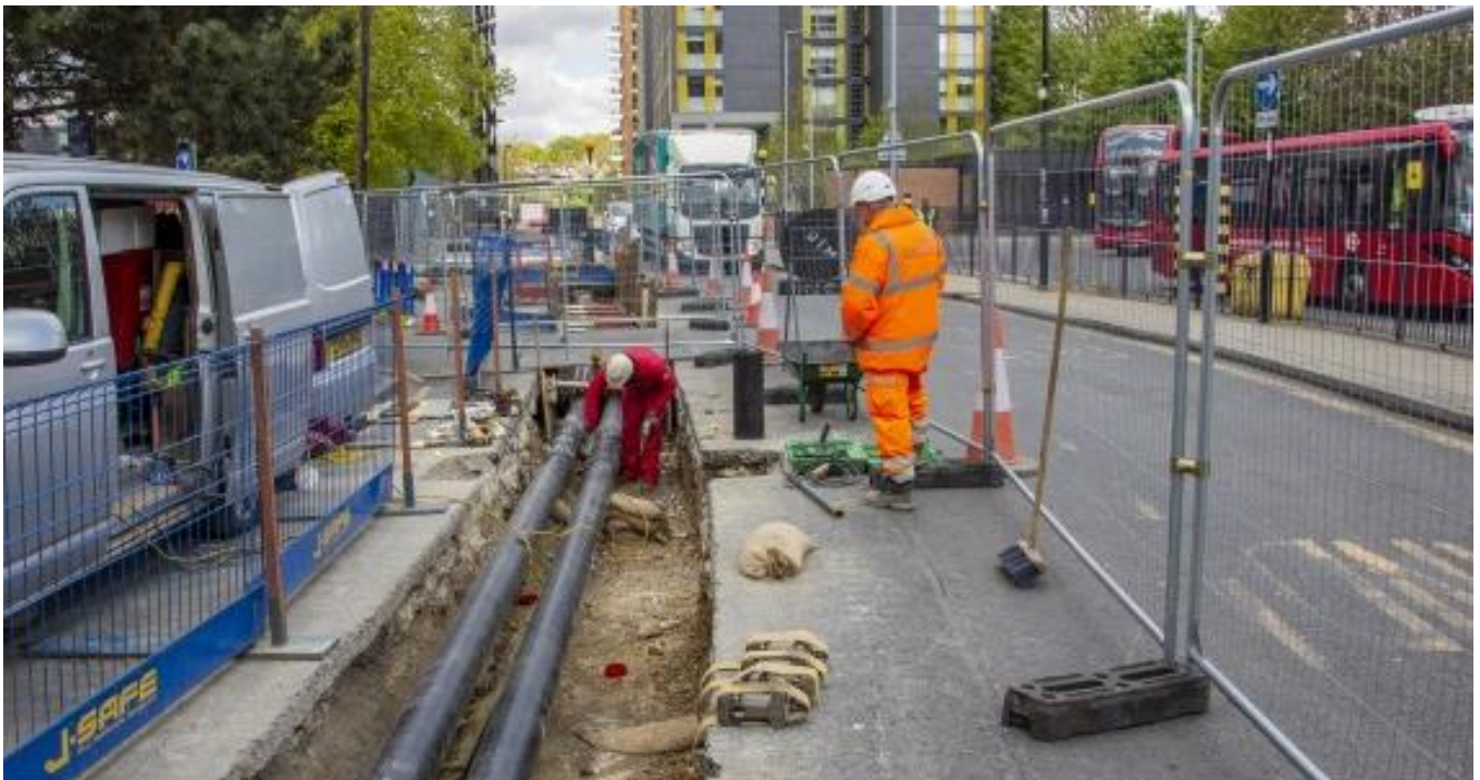
Image courtesy of CPC District Heating Ltd
